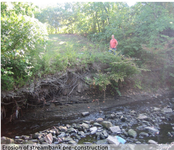
Erosion of streambank pre-construction
